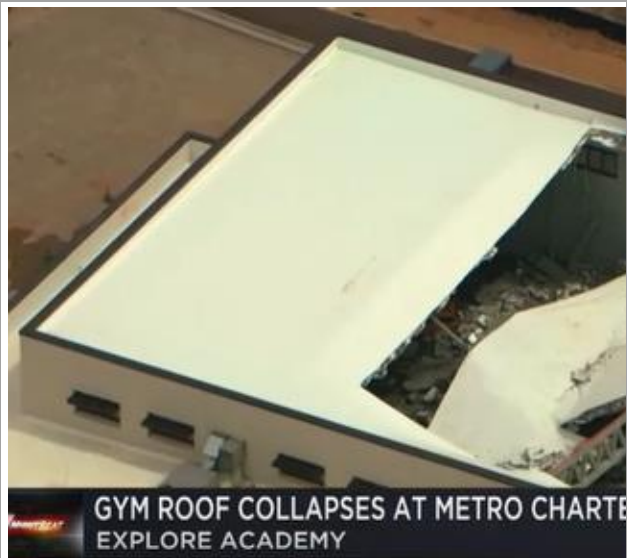
Albuquerque - damage under self-weight
